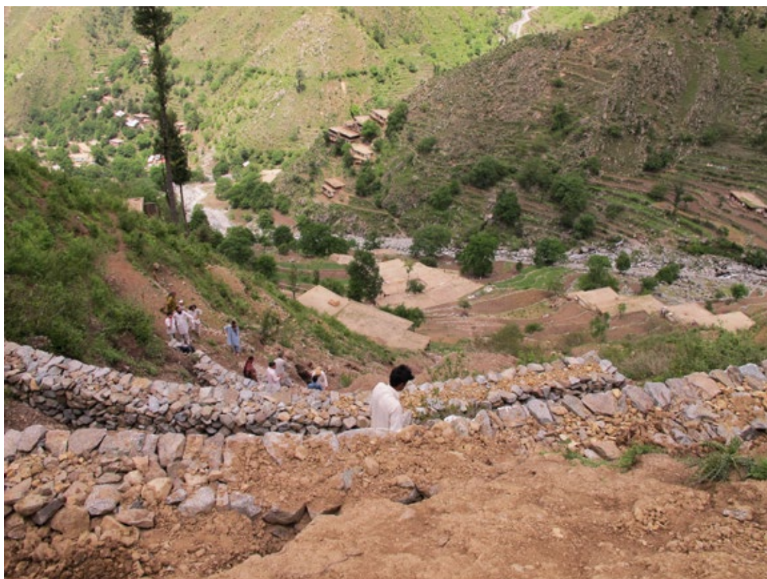
Figure 4: Slope stabilisation measures to mitigate flash floods in the Chail Valley in the Swat District of the north-western Pakistan, in the SDC and WFP Integrated food security and DRR programme. © SDC, Pakistan
